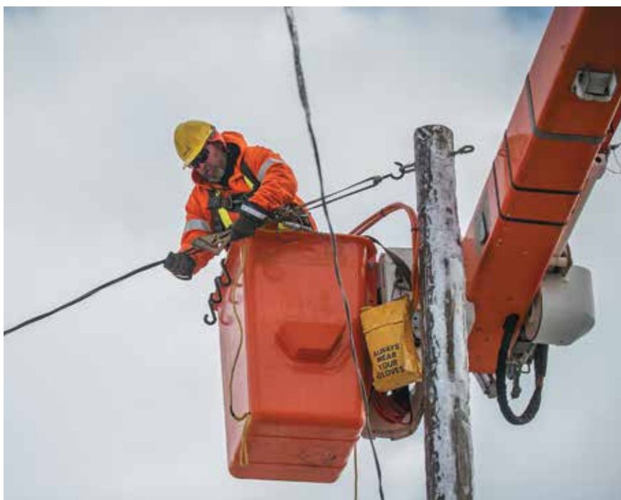
Our certified and specially-trained powerline technicians, like Bernie Harding (above), work day and night in all weather conditions to keep power on for Alectra Utilities customers.
