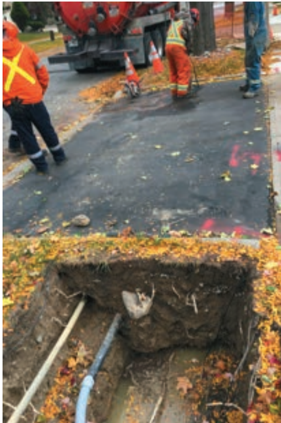
Shallow excavations like this one usually present less risks, however inaccurate locates can still lead to damages, as it happened in this case.
