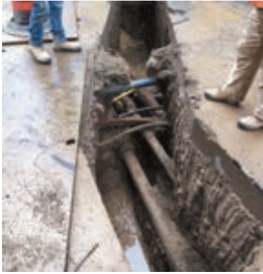
A few of these utilities were unknown and found while excavating.
