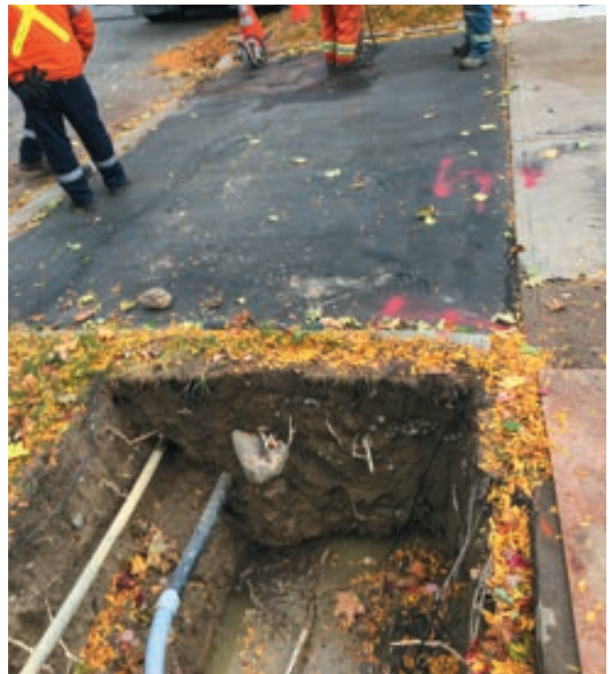
A few of these utilities were unknown and found while excavating. Read more about this story on Page 15.
